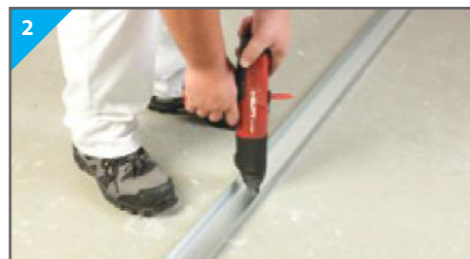
2 Determine and mark wall position and make allowance for openings. Fix Donn UltraSTEEL® Track at 600mm centres using suitable fixings.
